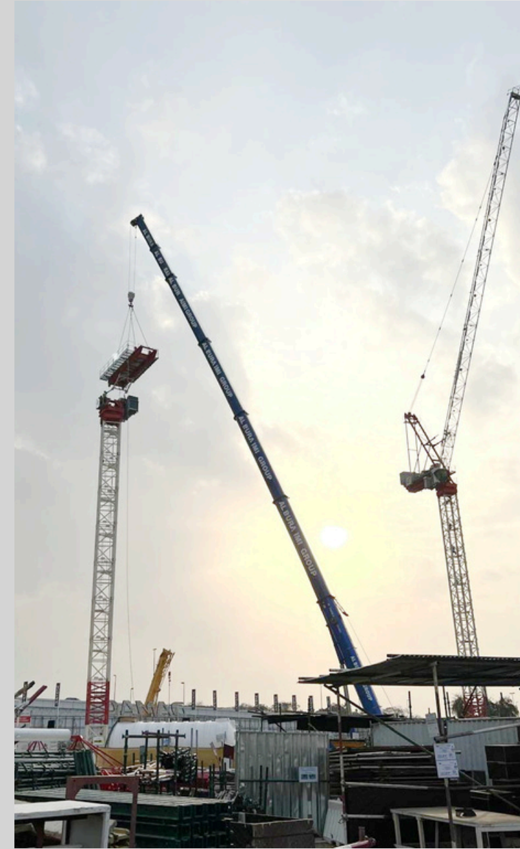
Hammer Head Tower Cranes
